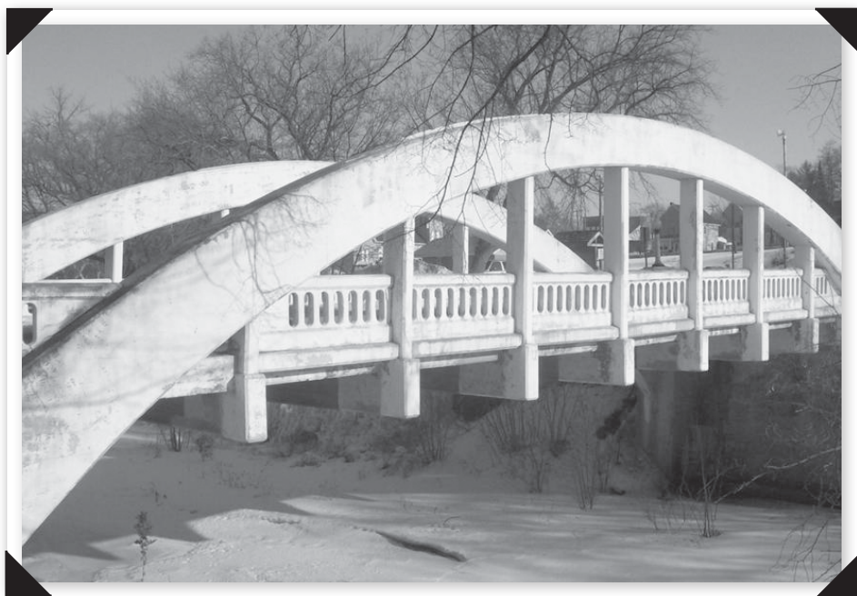
Marsh Rainbow Arch Bridge was built in 1916 by the Iowa Bridge Company at a cost of $13,950.
